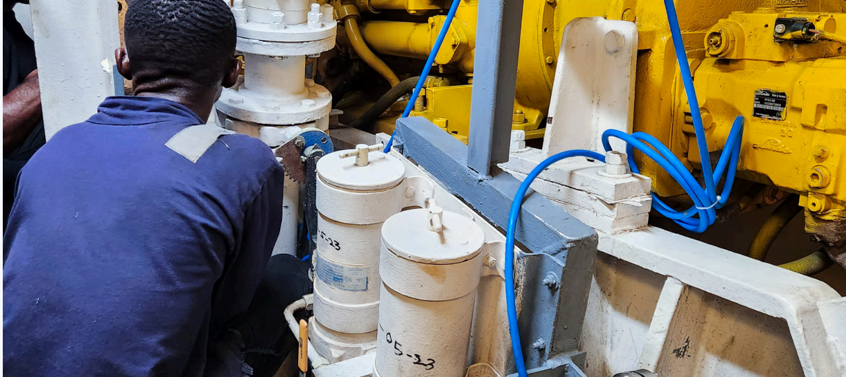
Coriolis flow meters on the fuel lines are needed for in-depth fuel control as part of a vessel monitoring system
